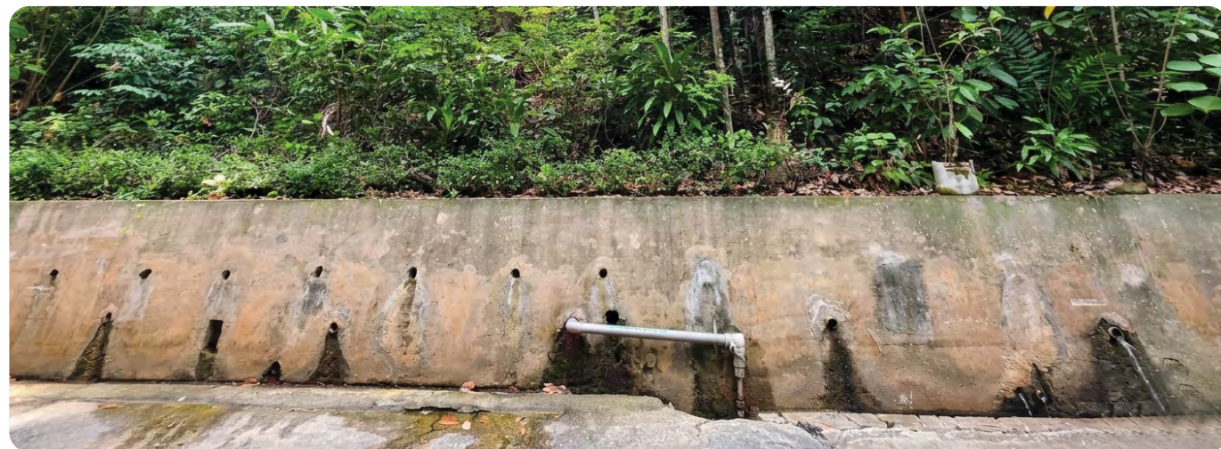
Spring water recovery system at AEON Mall Alpha Angle, redirecting natural flow from the adjacent jungle and collected for non-potable cleaning operations.
