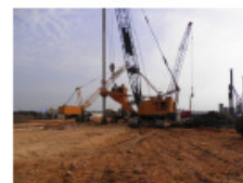
Bored Piling: Elevated terminal approach road for new airport in Sepang, Selangor
