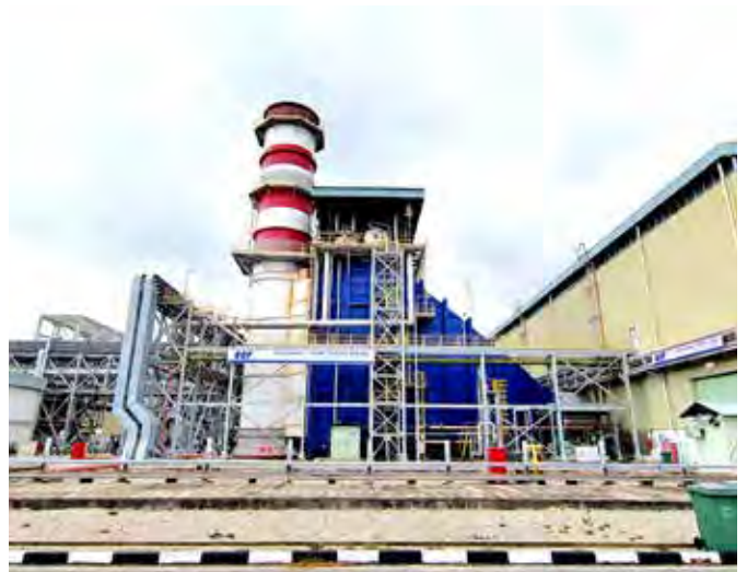
Segari Power Plant, Perak
