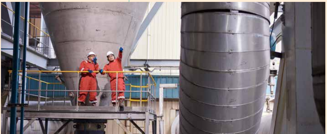
Reliability within our thermal plants were upheld through disciplined maintenance, strong asset management and enhanced technical and process controls that ensured smooth, stable daily operations.
