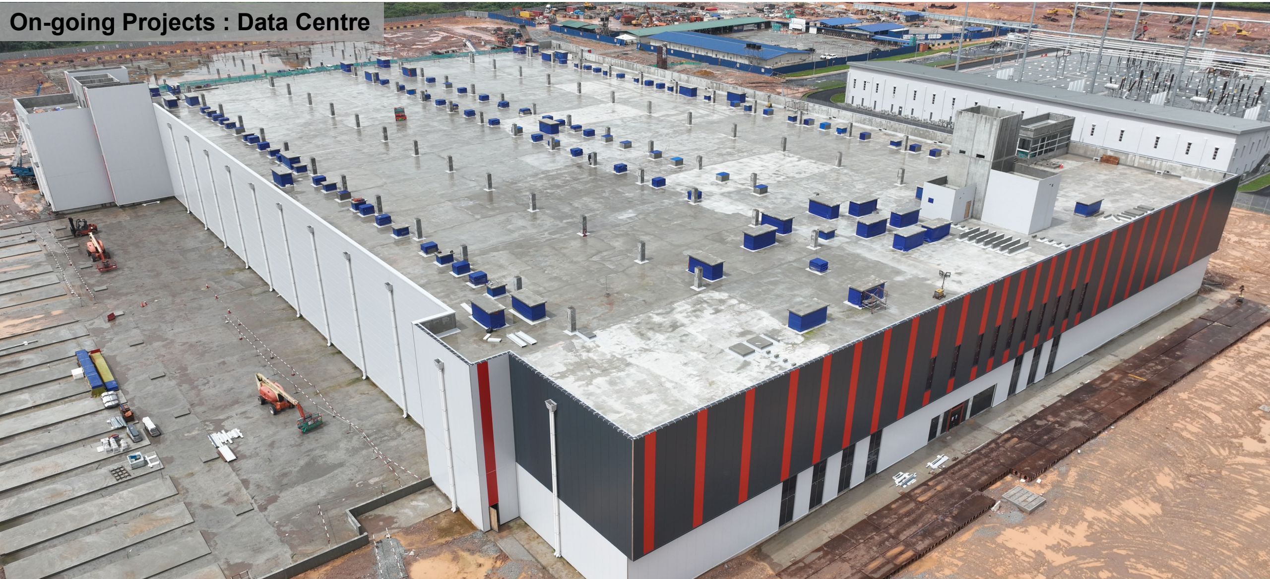
Data Centre at Sedenak, Johor
