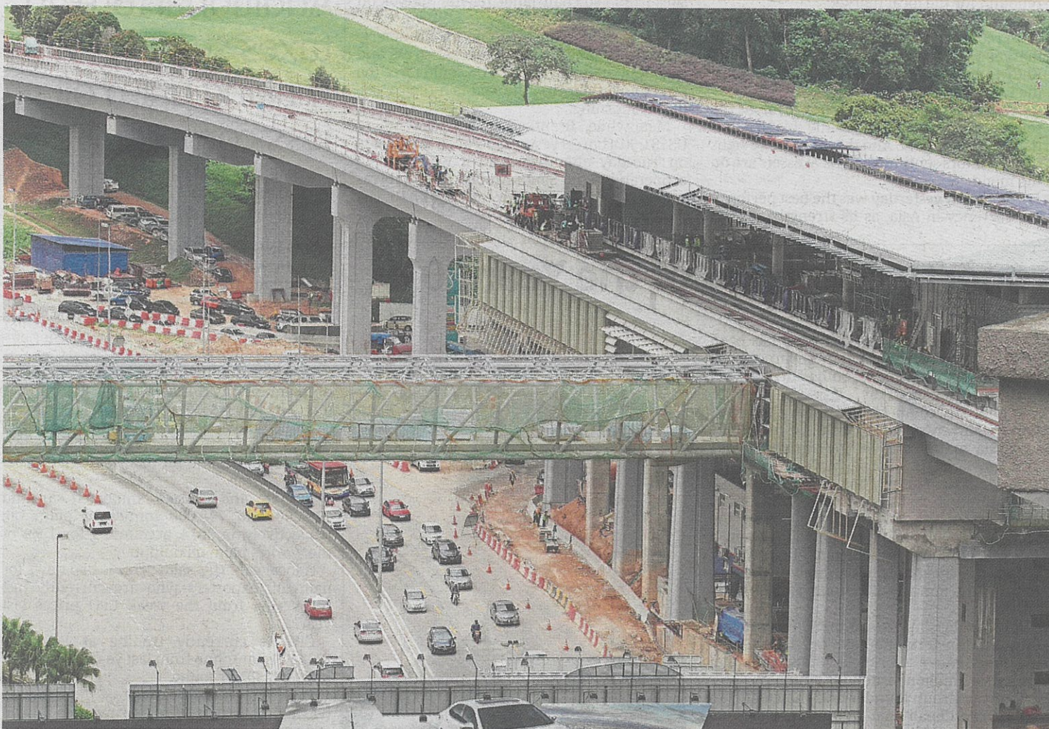
New station: The Phileo MRT station being constructed at Section 16, Petaling Jaya. The station is part of the MRT 1 line from Sungai Buloh to Kajang.
