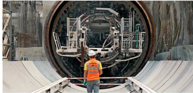
A filepic of a tunnel boring machine at the construction site of MRT2. While MMC-Gamuda has managed to retain the project, the underground cost reduction will still eat into margins. Photo by Bernama
