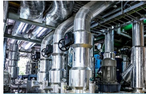
Mechanical, Electrical and Plumbing Services
