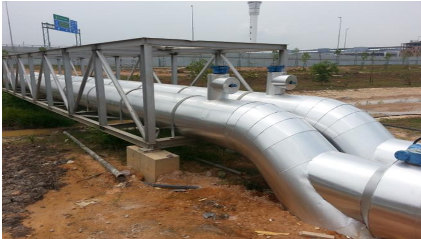
KLIA Chilled Water
