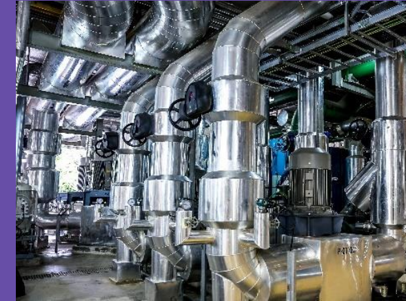
Mechanical, Electrical and Plumbing Services
