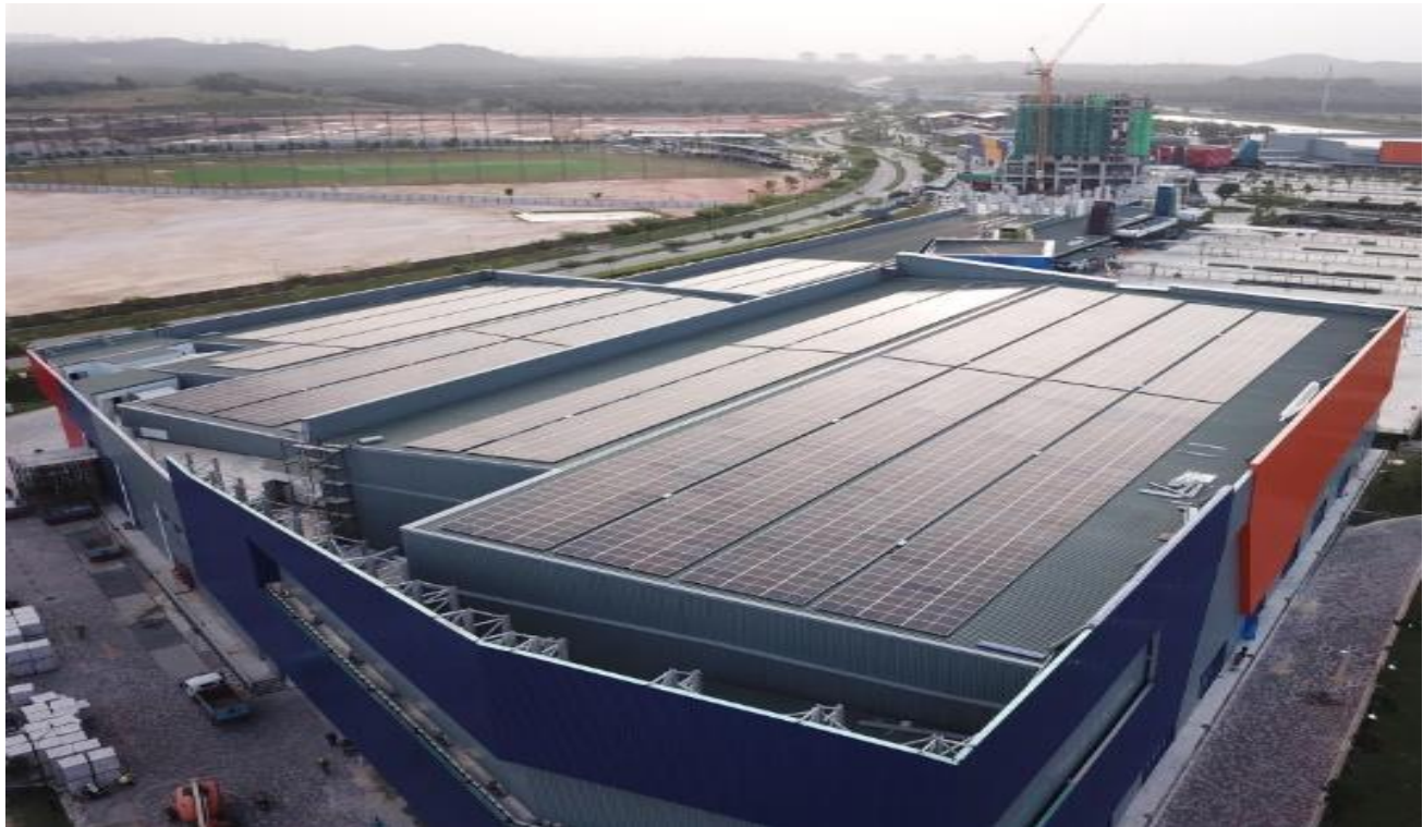
Roof Top Solar – Sunway Iskandar
