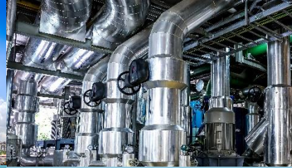
Mechanical, Electrical and Plumbing Services
