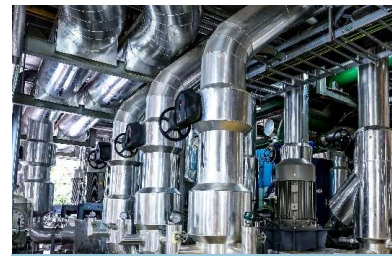
Mechanical, Electrical and Plumbing Services
