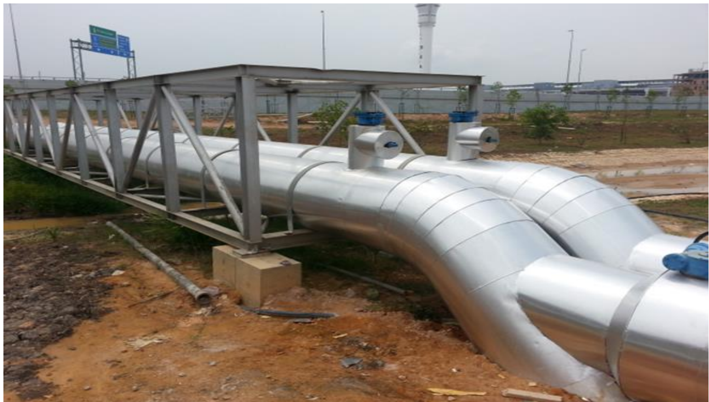
KLIA Chilled Water
